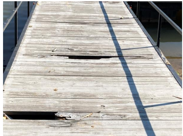
Staghorn Fishing Dock Boards have rotted.
